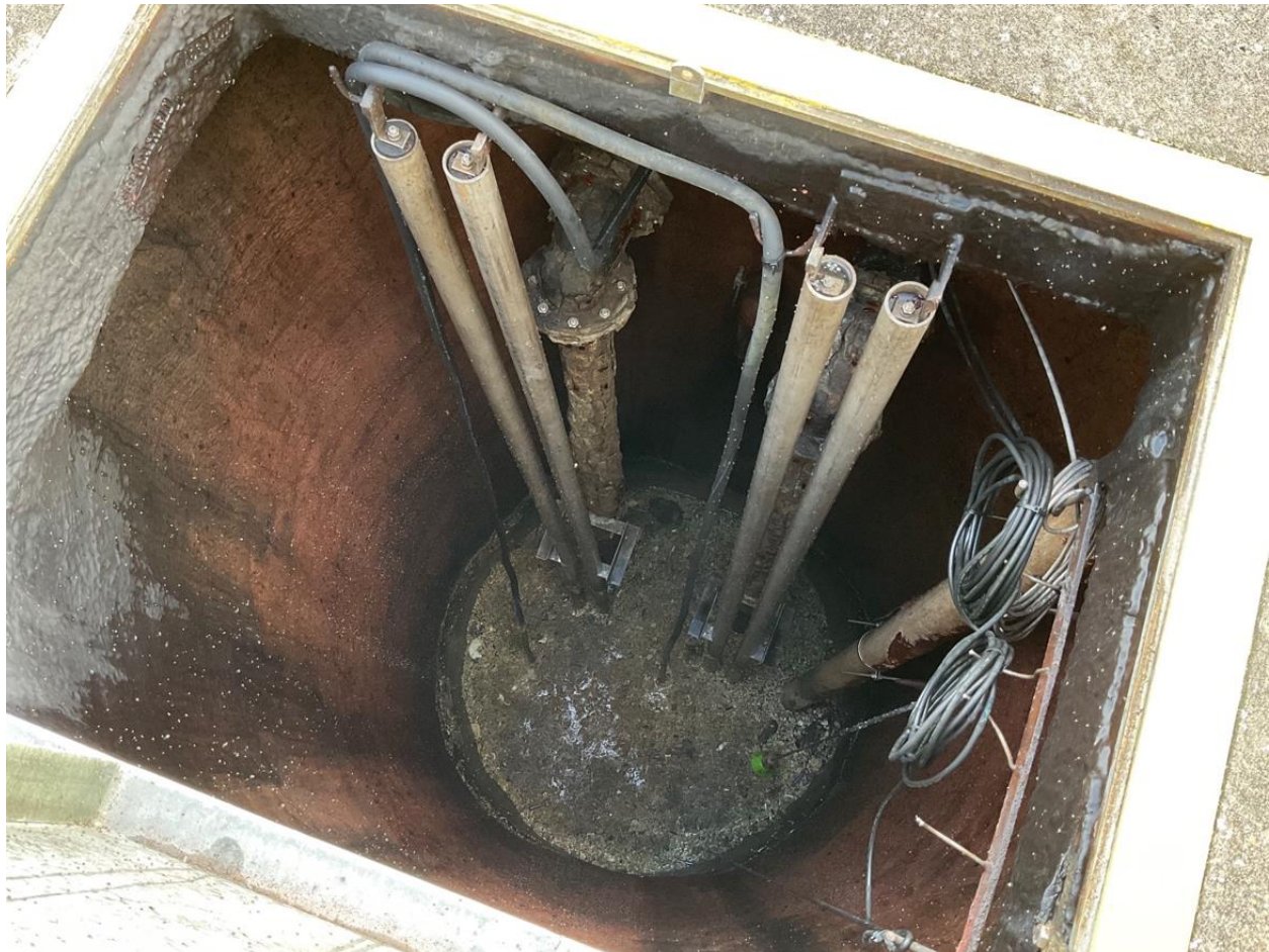
FIGURE 4-8: LIFT STATION 6 WET WELL
