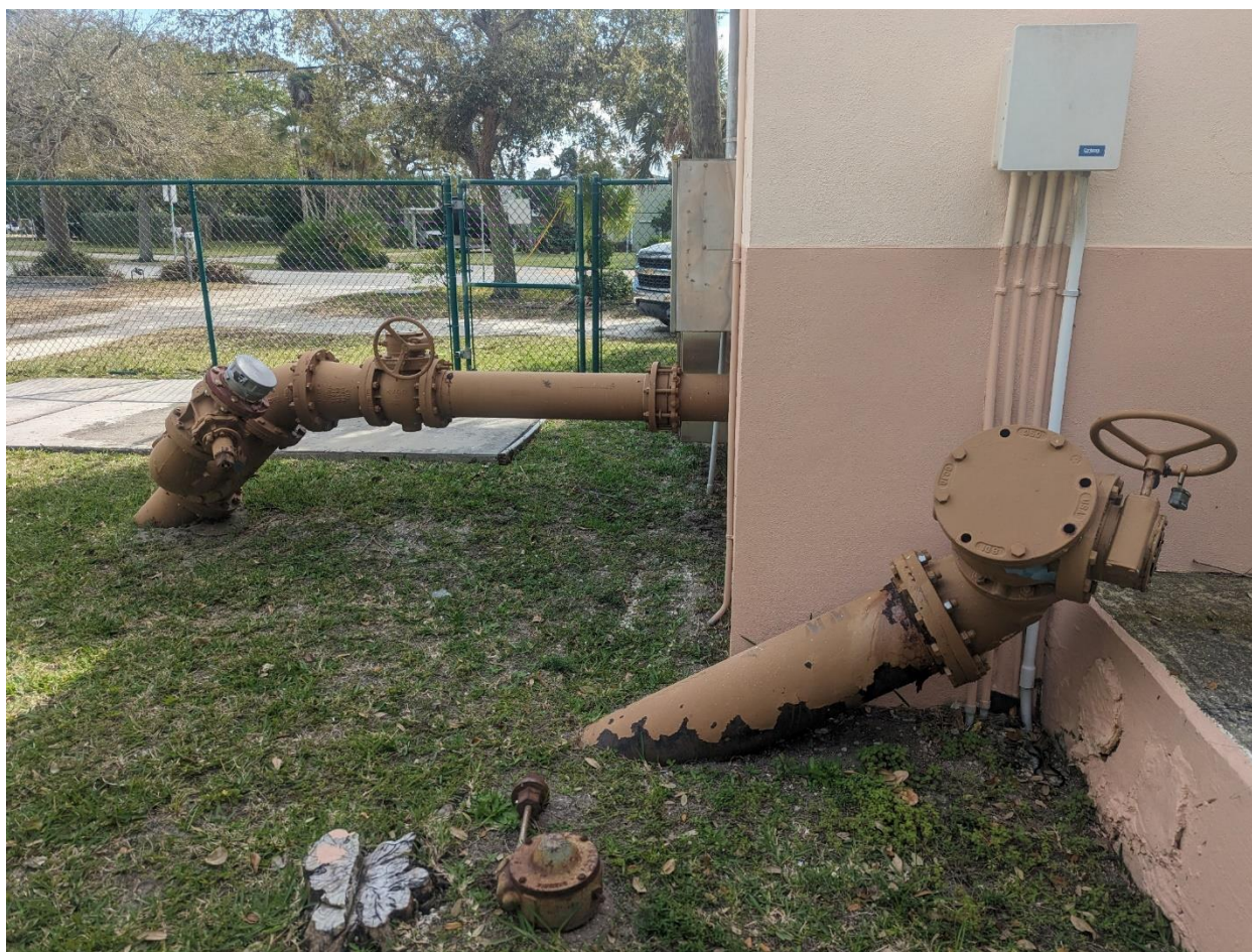
FIGURE 4-5: LIFT STATION 4 BYPASS VALVE
