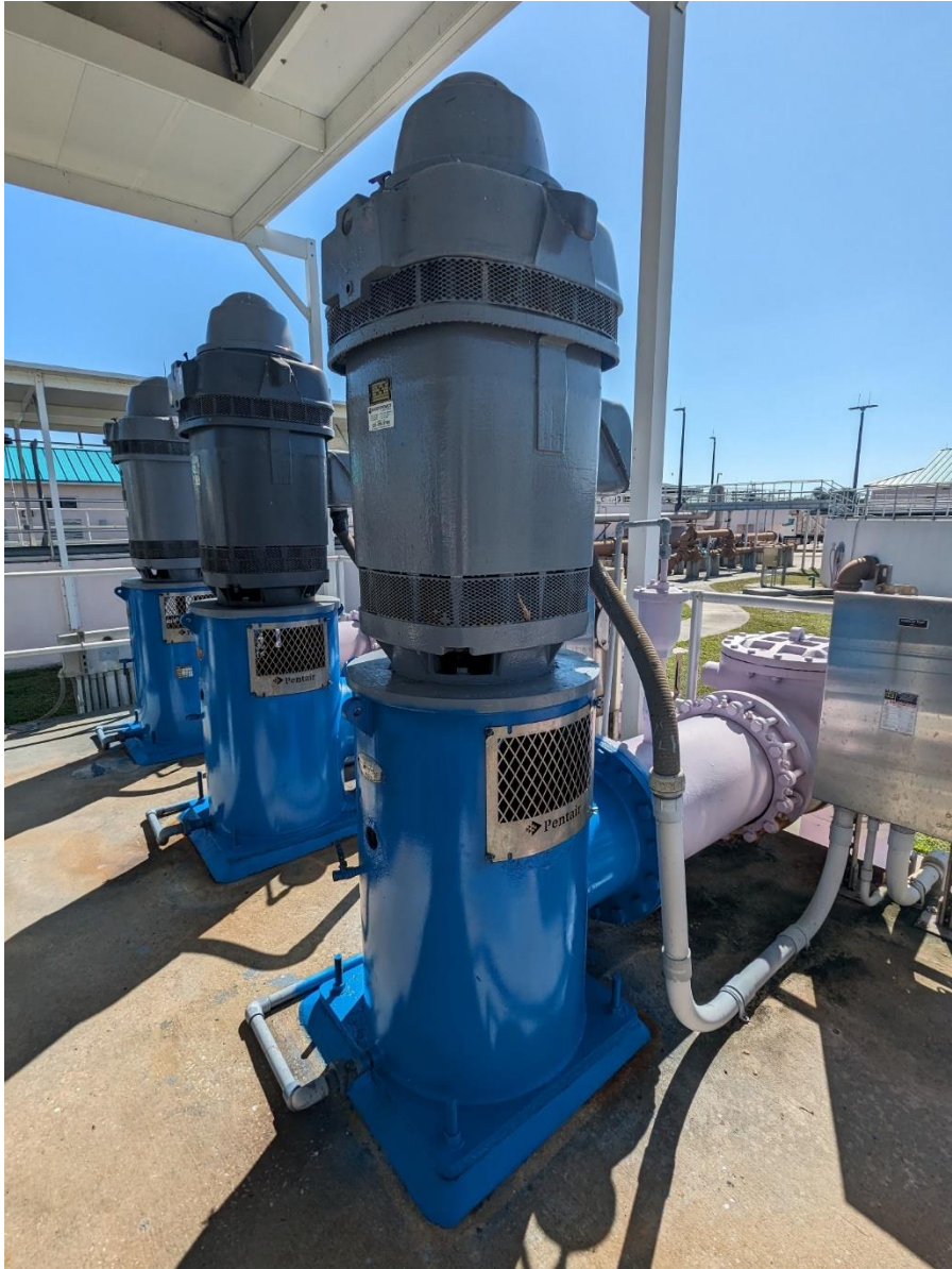
FIGURE 4-32: WRF REUSE TRANSFER PUMPS
