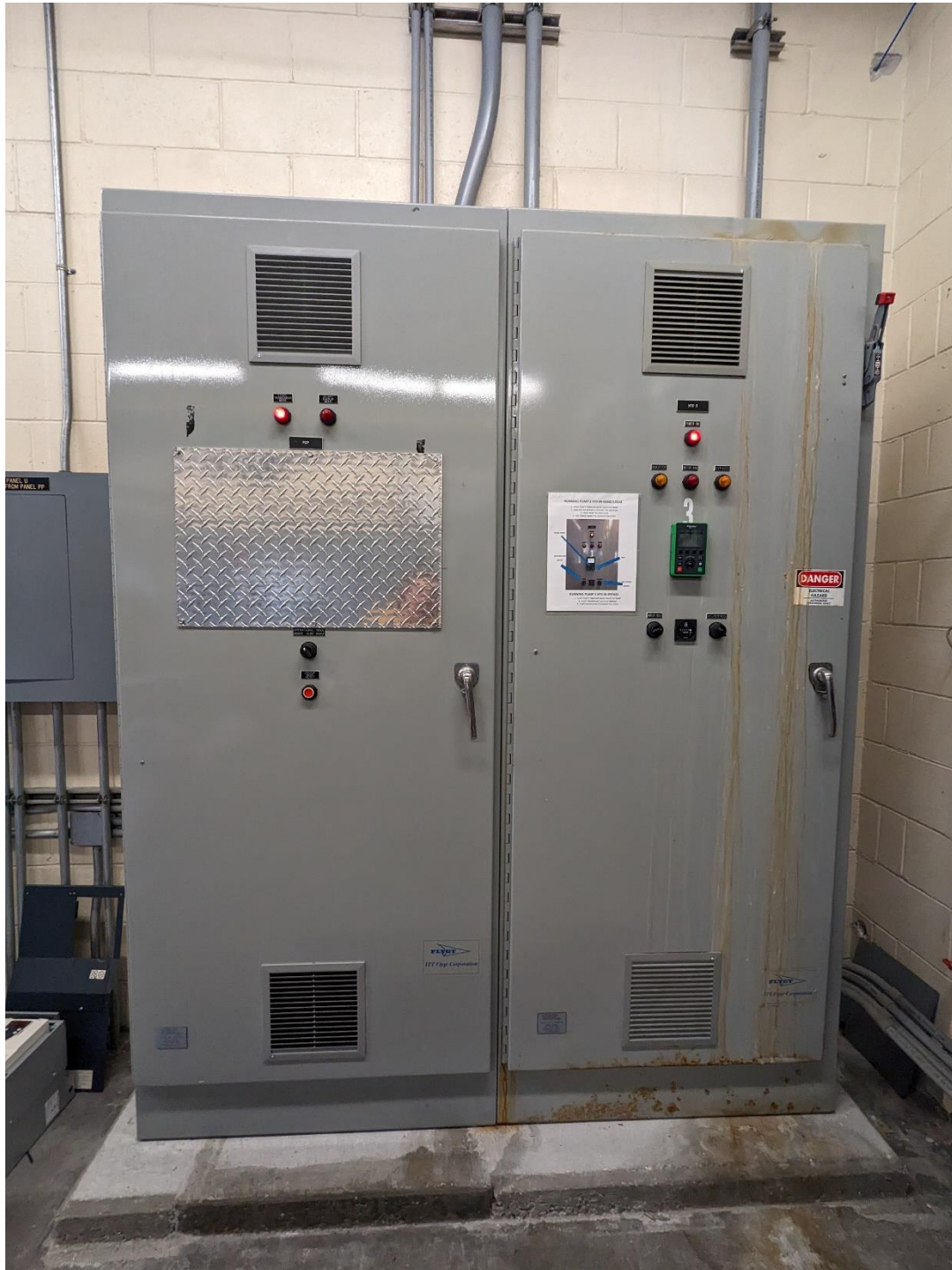
FIGURE 4-7: LIFT STATION 5 PCP AND VFD 5
