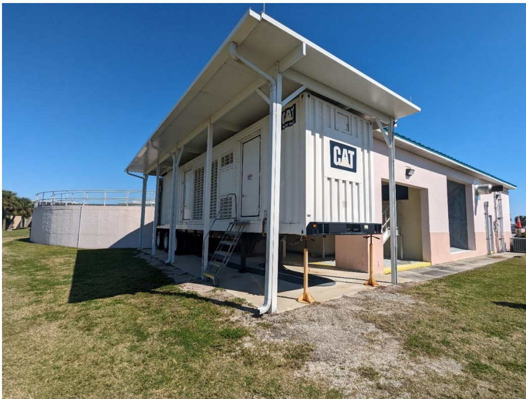
FIGURE 4-30: WRF EMERGENCY GENERATOR 2
