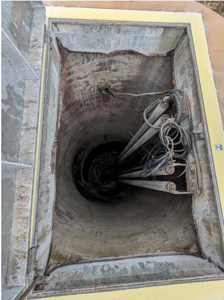
FIGURE 4-14: LIFT STATION 10 WET WELL
