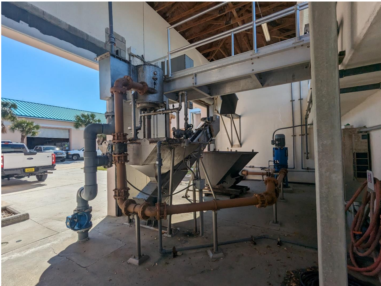
FIGURE 4-27: WRF GRIT REMOVAL EQUIPMENT
