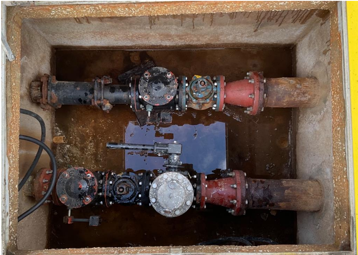
FIGURE 4-9: LIFT STATION 6 VALVE VAULT
