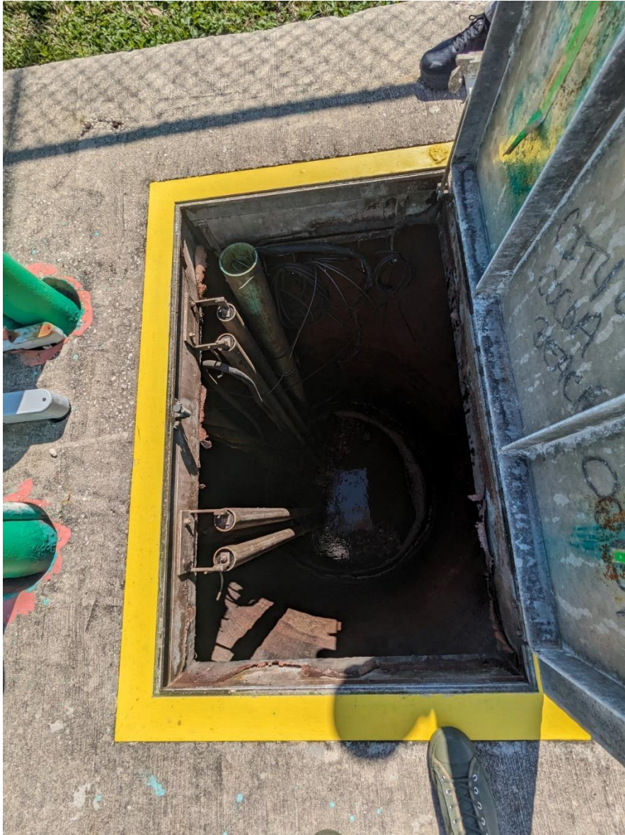
FIGURE 4-11: LIFT STATION 8 WET WELL
