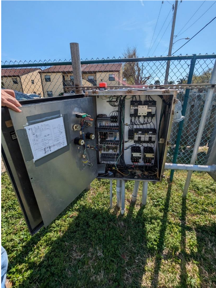
FIGURE 4-13: LIFT STATION 8 CONTROL PANEL
