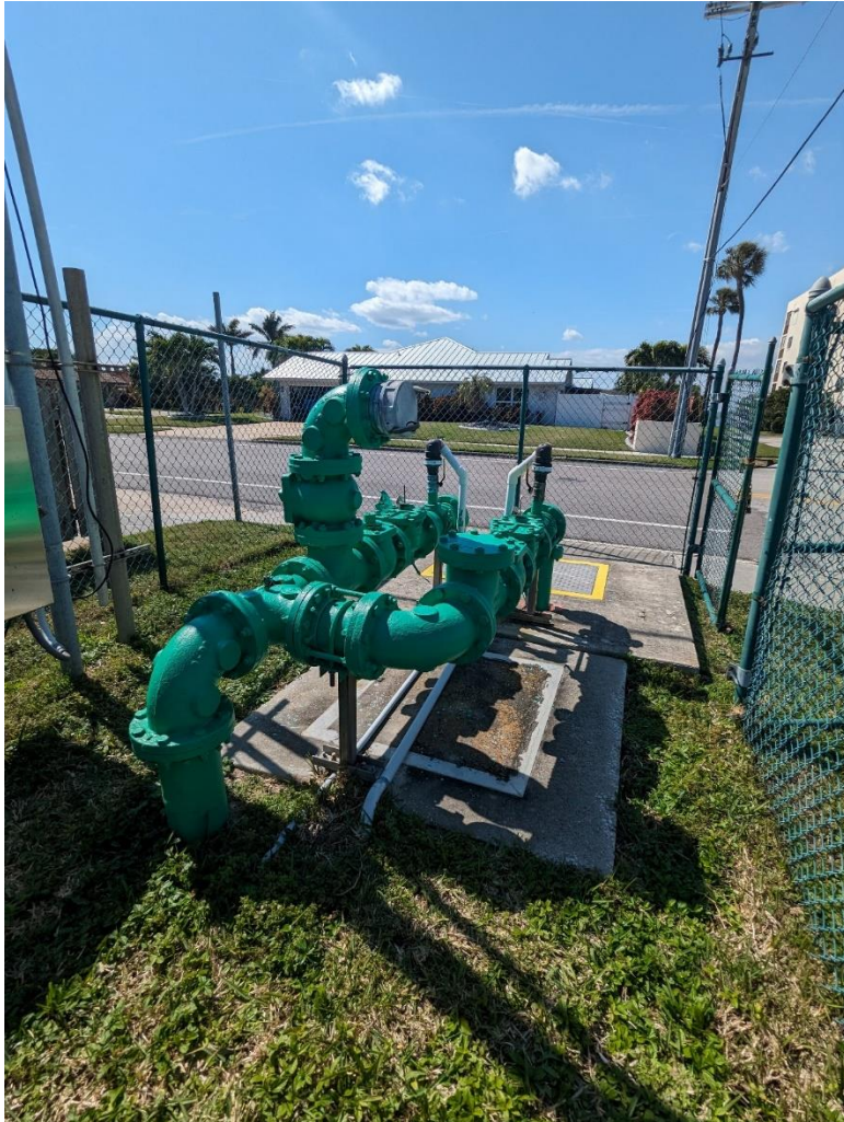
FIGURE 4-12: LIFT STATION 8 ABOVE GRADE DISCHARGE VALVES
