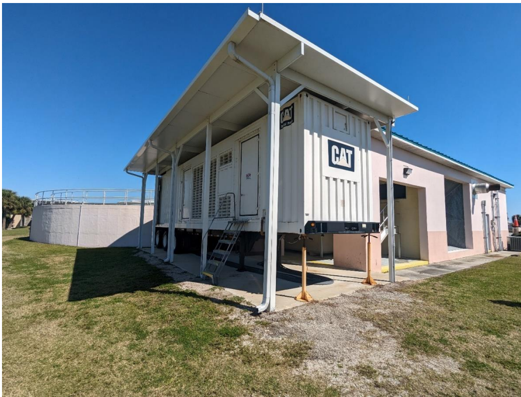
FIGURE 4-30: WRF EMERGENCY GENERATOR 2
