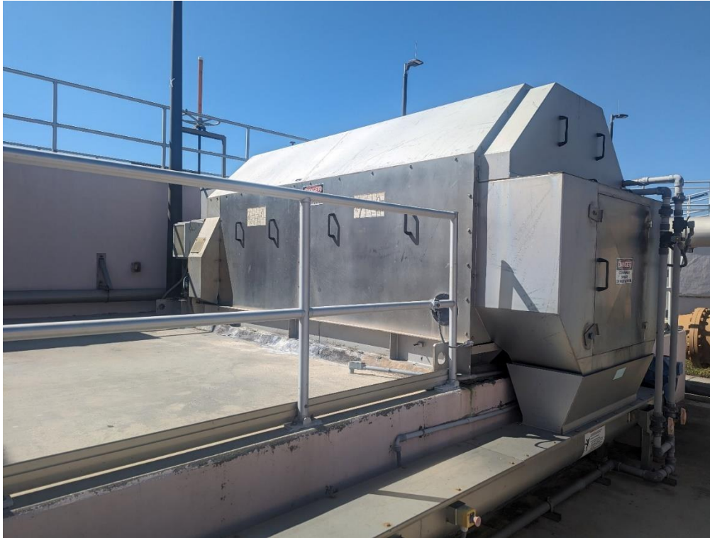
FIGURE 4-34: WRF DRUM SCREENS
