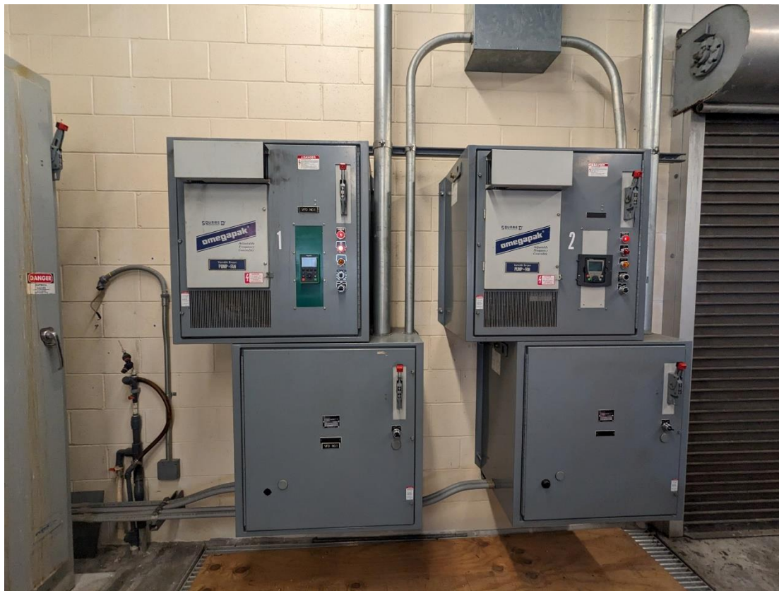
FIGURE 4-6: LIFT STATION 5 VFDS 1-4
