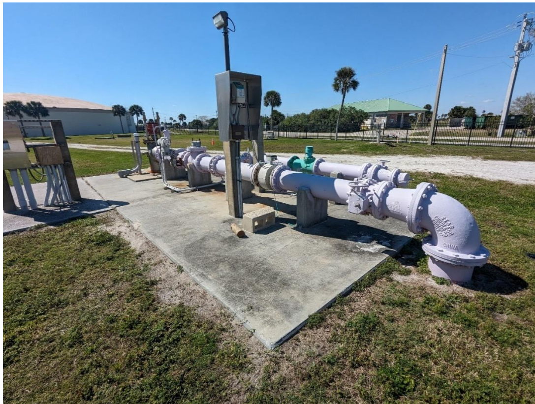
FIGURE 4-31: INJECTION WELL ABOVE GROUND PIPING
