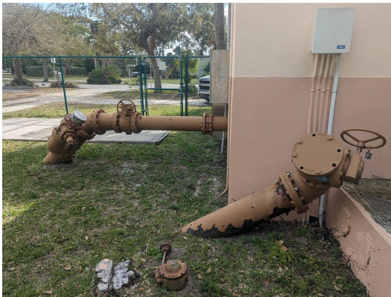
FIGURE 4-5: LIFT STATION 4 BYPASS VALVE
