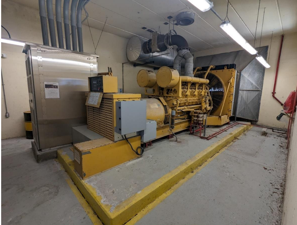
FIGURE 4-29: WRF EMERGENCY GENERATOR 1
