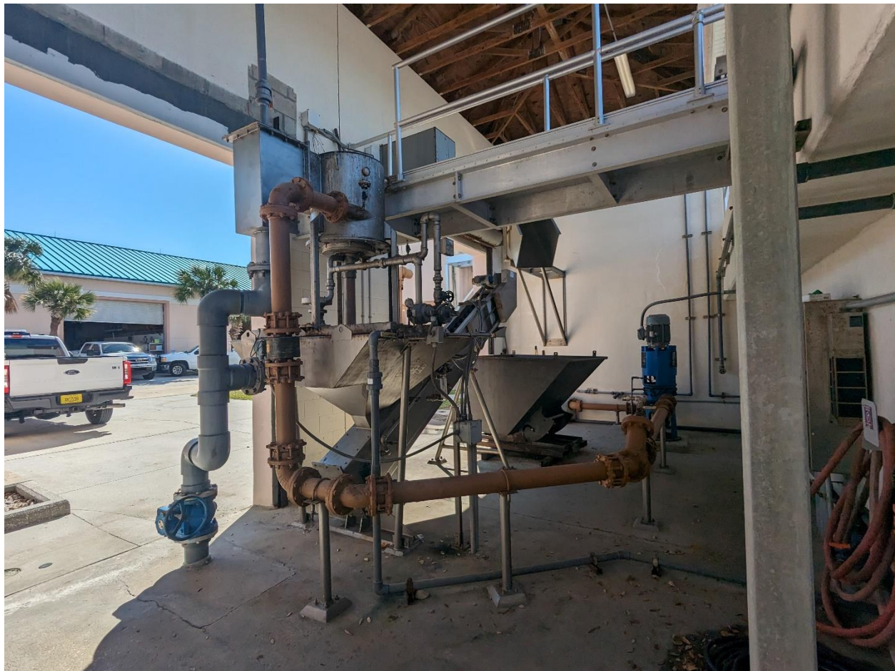
FIGURE 4-27: WRF GRIT REMOVAL EQUIPMENT
