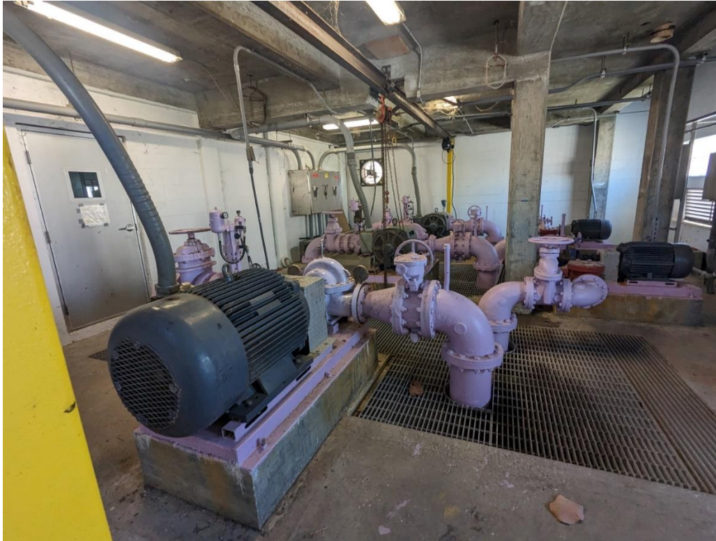
FIGURE 4-33: WRF REUSE HIGH SERVICE PUMPS
