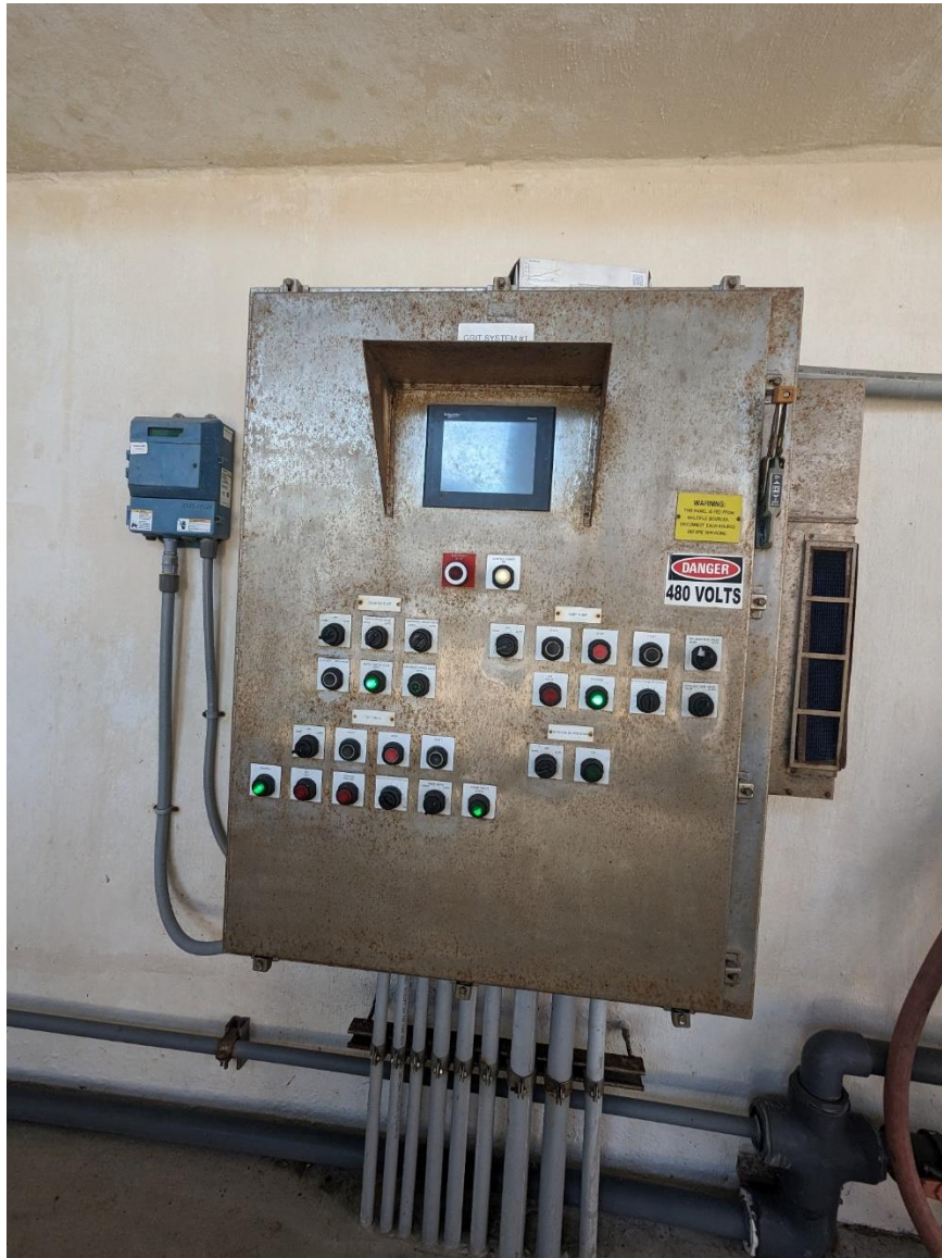
FIGURE 4-28: GRIT REMOVAL SYSTEM CONTROL PANEL
